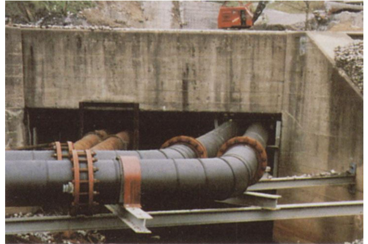
16-inch-diameter drainage pipes designed to convey water from mine shaft to existing treatment ponds.
