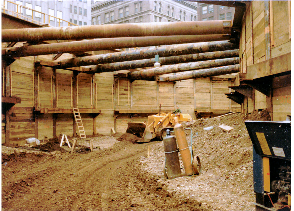
Braced excavation for construction of the Gateway Center subway station in Pittsburgh.
