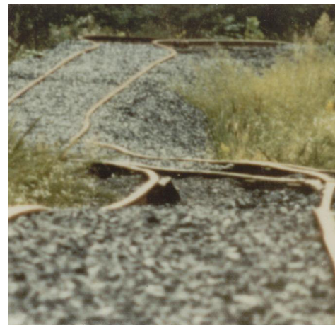
Observed offset in site railroad track caused by movement of slope.
