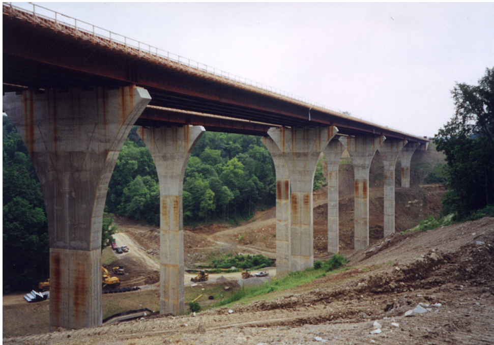
Dual bridge structures at Section 52-E of the Mon Fayette Expressway under construction.
