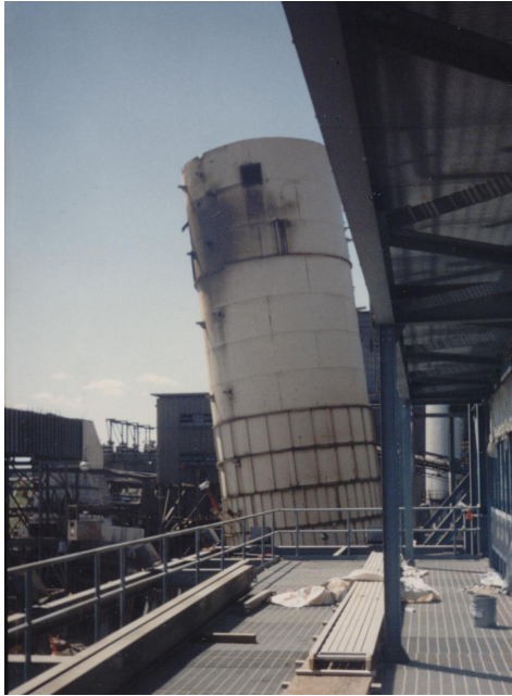
Storage tank exhibiting tilt resulting from foundation failure caused by collapse of subgrade cooling pipes.
