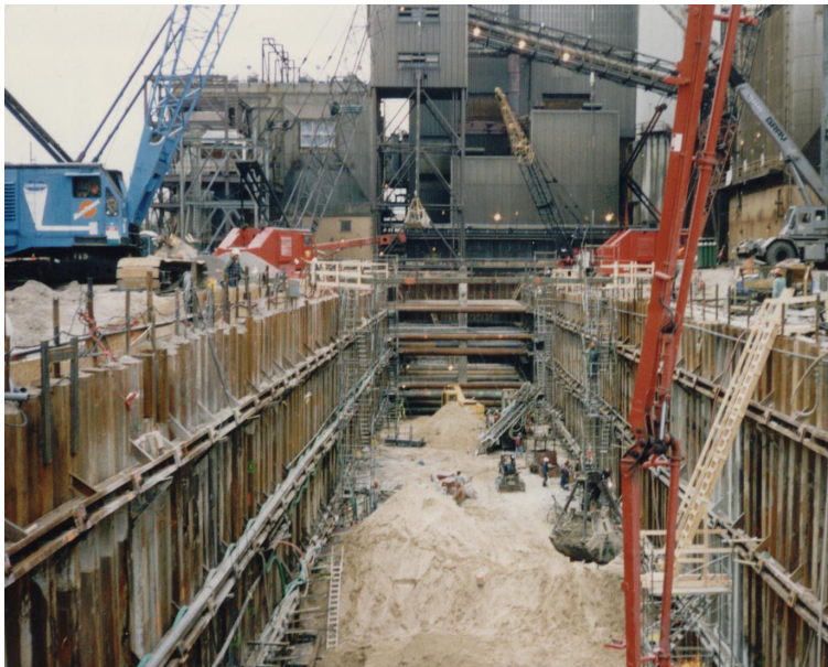
Sheet pile wall used for ground support during replacement of failed 14-foot-diameter cooling pipes located 60 feet below grade.
