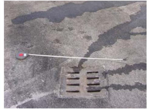
Typical storm drain leading to a dry well at the Aviano Air Base.
