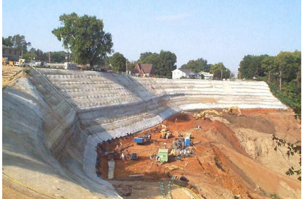
150-foot-high bluff situated along the Mississippi River during construction of a 95,000-square-foot stabilization system that incorporates soil nails and prestressed soil anchors.
