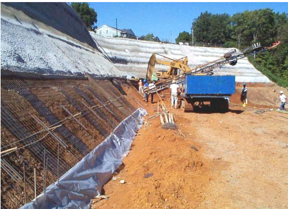
Drilling for installation of one of over 1,500 soil nails used in the stabilization system.
