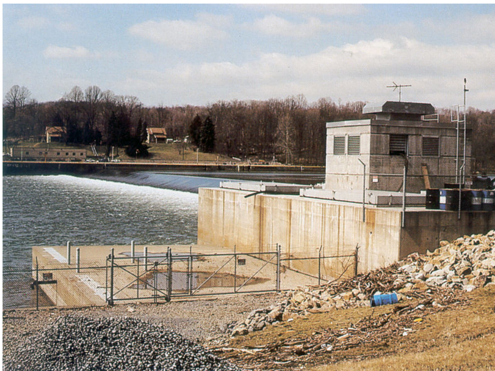
Completed 12-MW, low-head hydroelectric generation plant on the Allegheny River.
