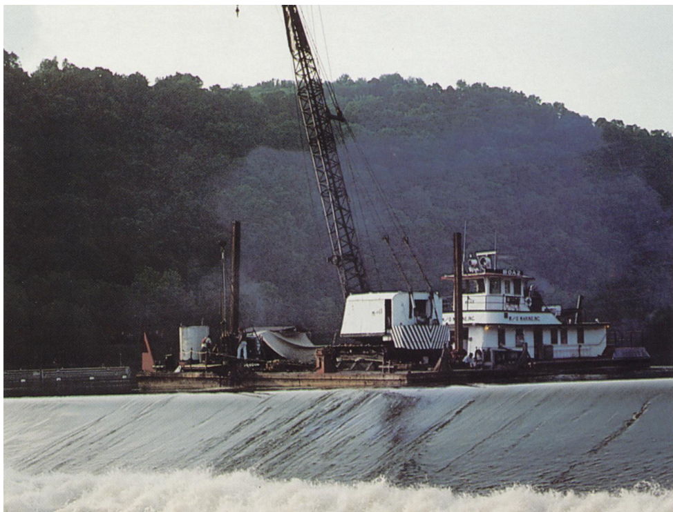
Drilling conducted from barge in the Allegheny River to obtain core samples from a concrete dam and samples of subsurface foundation soils.
