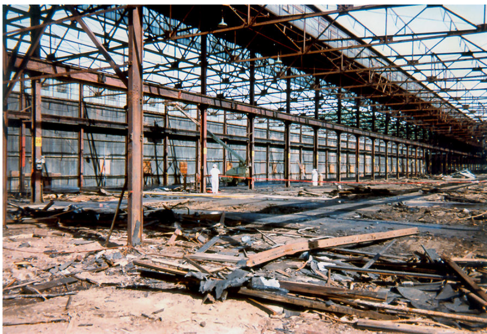
Asbestos-containing and deteriorated building materials were removed from warehouse structures, which were subsequently rehabilitated as part of redevelopment.
