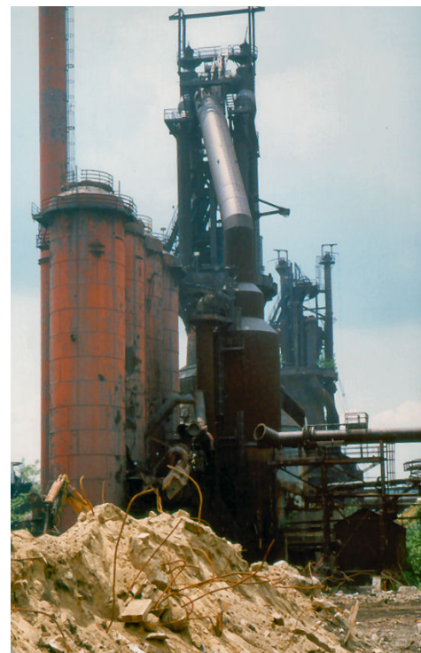
Scrap steel from demolition at this site was used to offset environmental remediation costs.
